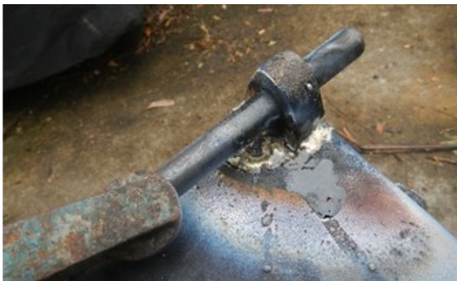
Photo 2 - 75% OK job – thankfully no photos post the subsequent "improvement" attempt exist .
